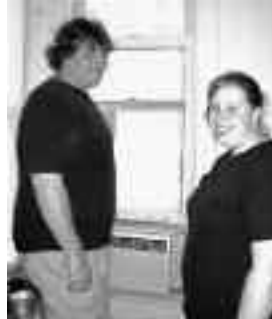
Service Providers, Tim Stewart and Jana Lakebrink, install an air conditioning unit in the home of an at-risk client.
